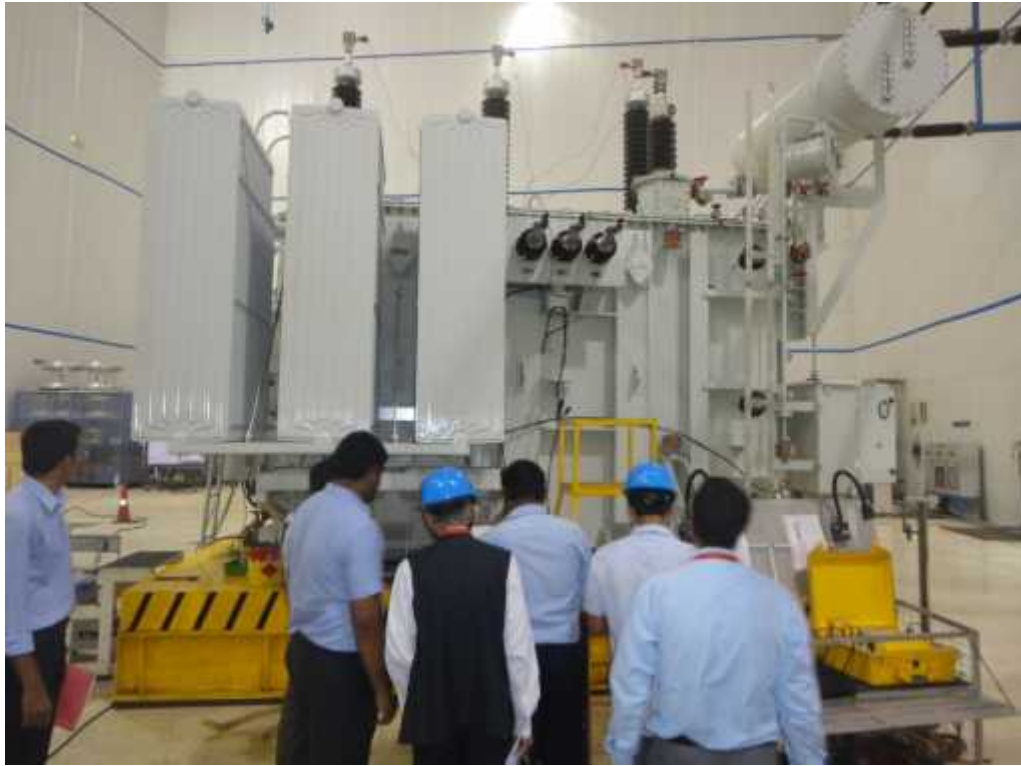
Inspection of Transformer
